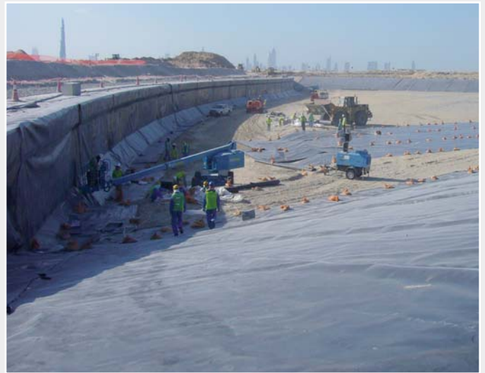
A small section of the enormous installation. On the left in the background is the «Burj Dubai».
